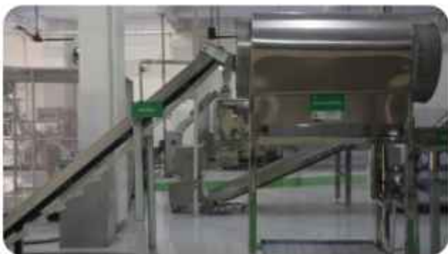
RTE Pilot Plant
